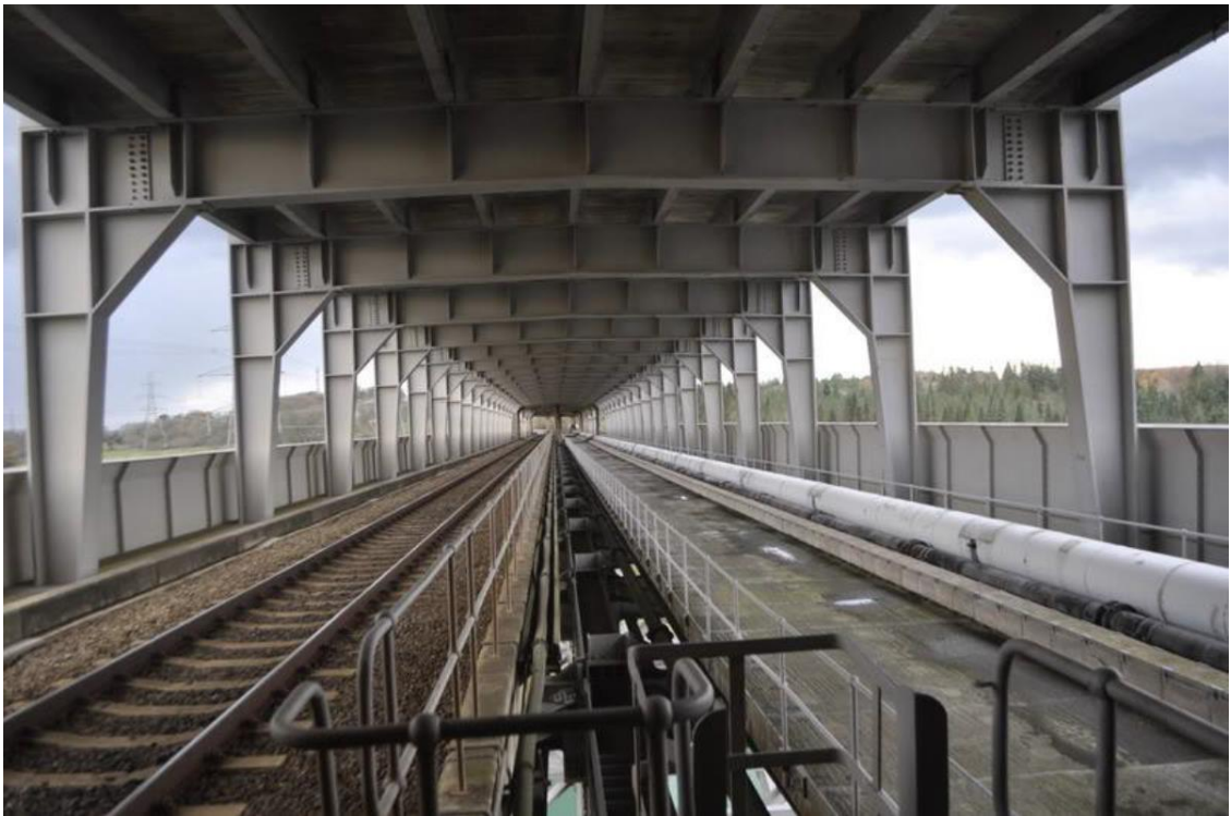
Figure 1-1 Britannia Bridge lower deck showing the proximity of the Bangor to Llanfair AC circuit cables to the railway.
