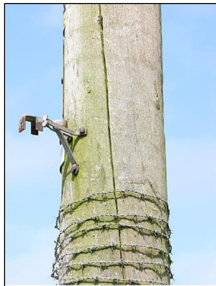
Figure 12 - AT091 Splitting at Middle of Pole
