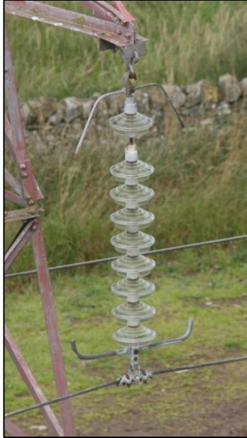
Figure 5 - U052 Broken Insulator
