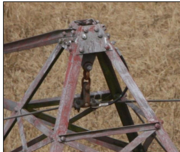
Figure 8 - U050 Corroded/Worn Earth-wire Fitting
