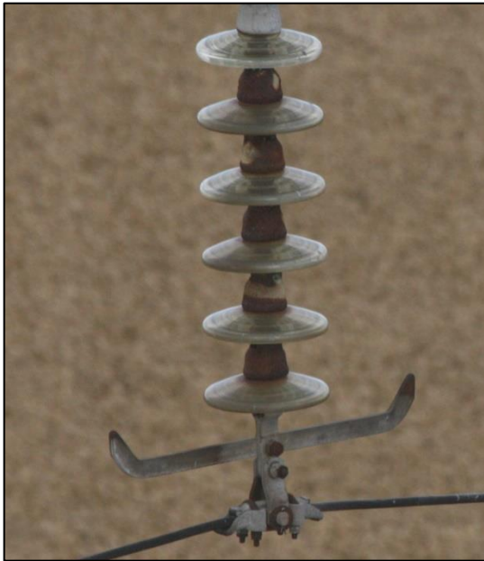
Figure 9 - AT158 Severely Corroded Insulators
