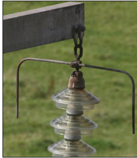
Figure 10 - AT115 Severely Worn Fittings
