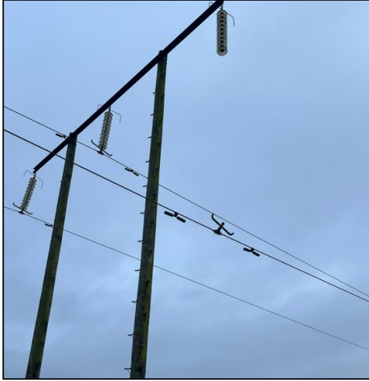
Figure 13 - Low Hanging Live Conductors AT092
