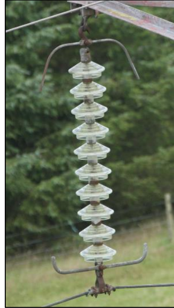
Figure 6 - U010 Corroded/Worn Fittings
