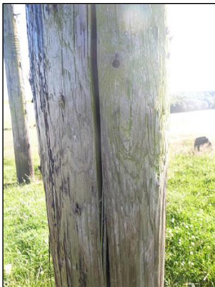
Figure 11 - AT028 Splitting at Base of Pole
