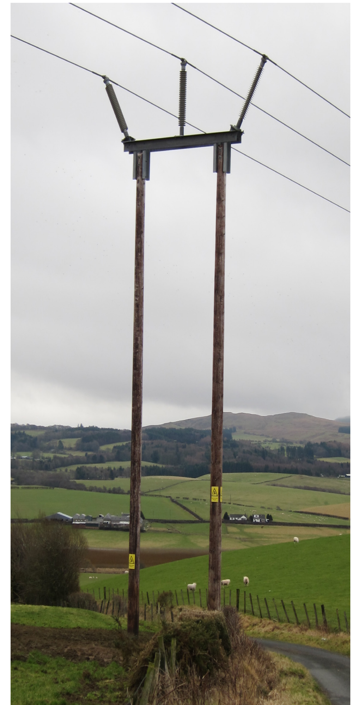
Typical Trident 132kV 'H' wood pole
