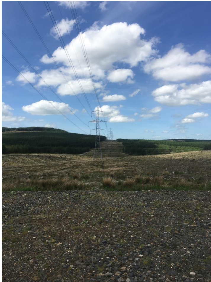
View of the 275kV WA Overhead Line between Coylton and New Cumnock substations
