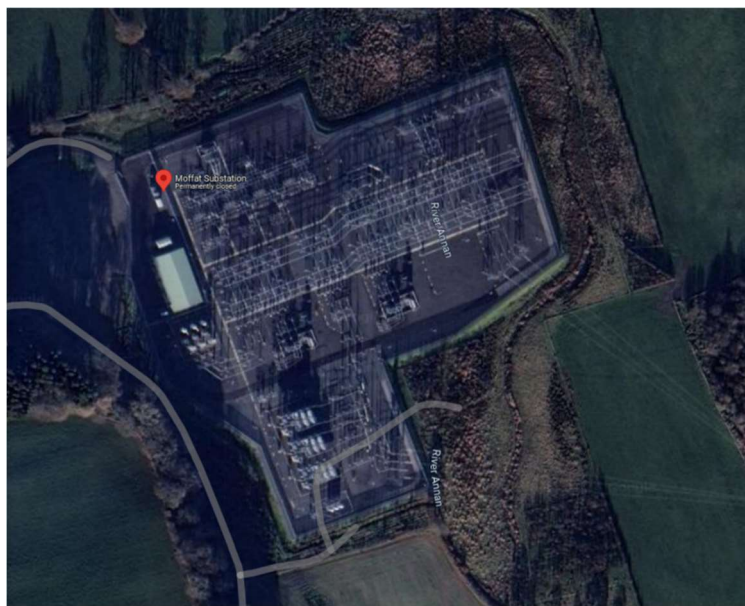
Figure 1: Moffat 400kV substation
