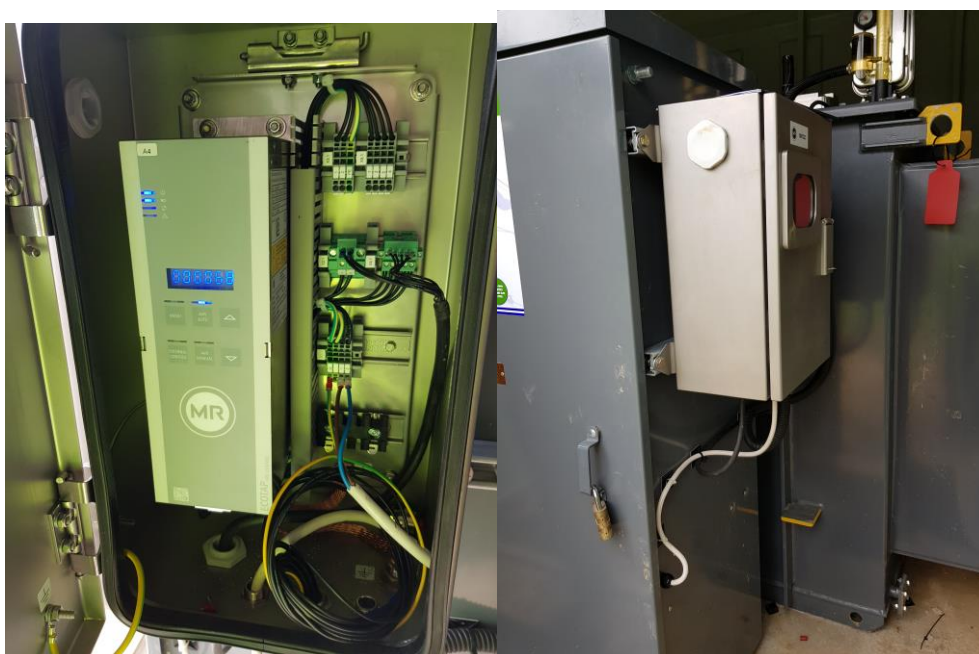
Markle Mains Farm – Installed On-Load Tap Changing Secondary Transformer
