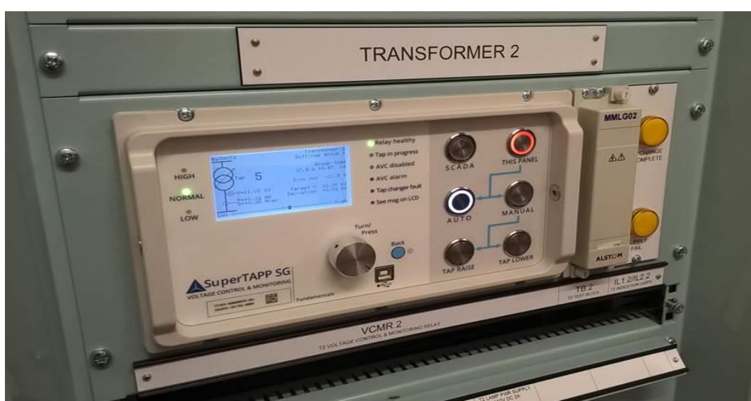
Ayton Primary installed SuperTapp+ AVC Scheme
