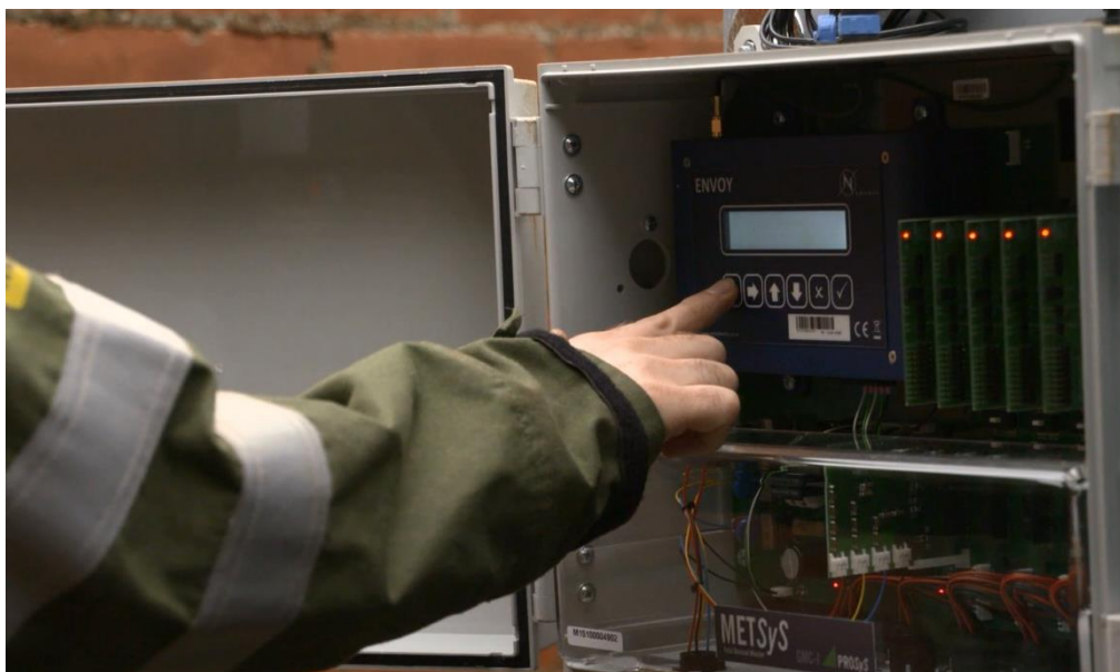
Figure 20: LV Secondary Substation Monitor
