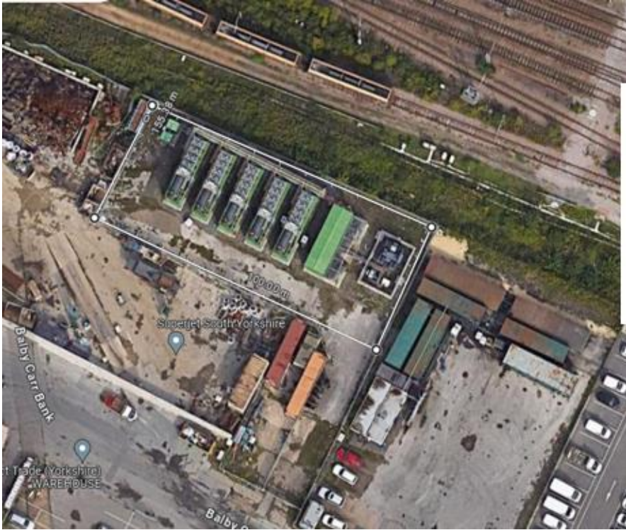
Battery Storage Example
