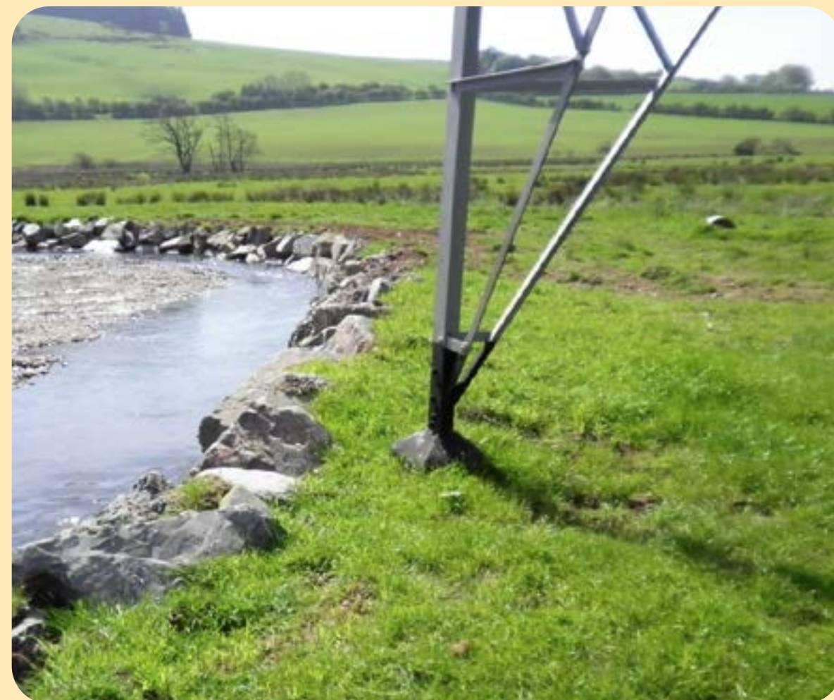
Climate change causing river bank erosion, putting transmission tower at risk
