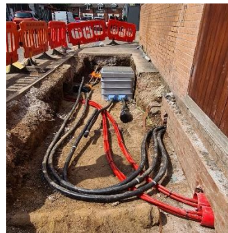
Cabling outside the substation
