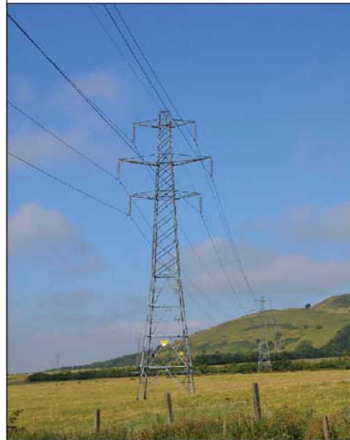
Component parts of 132kV Steel Lattice Tower L4: Glenlee to Tongland
