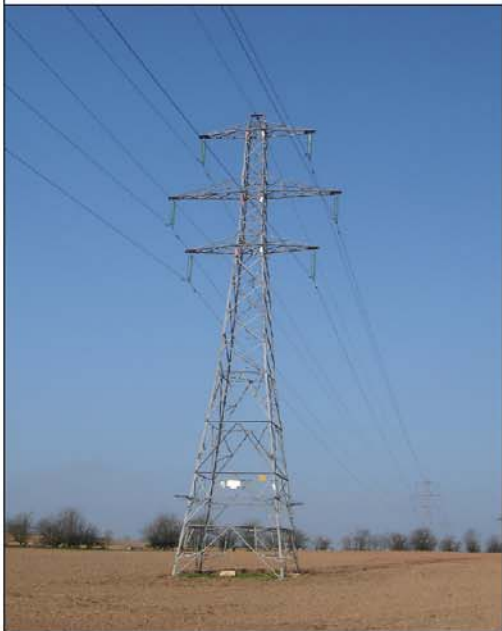
Component parts of 132kV Steel Lattice Tower L7: Polquhanity to Kendoon, and Kendoon to Glenlee.
