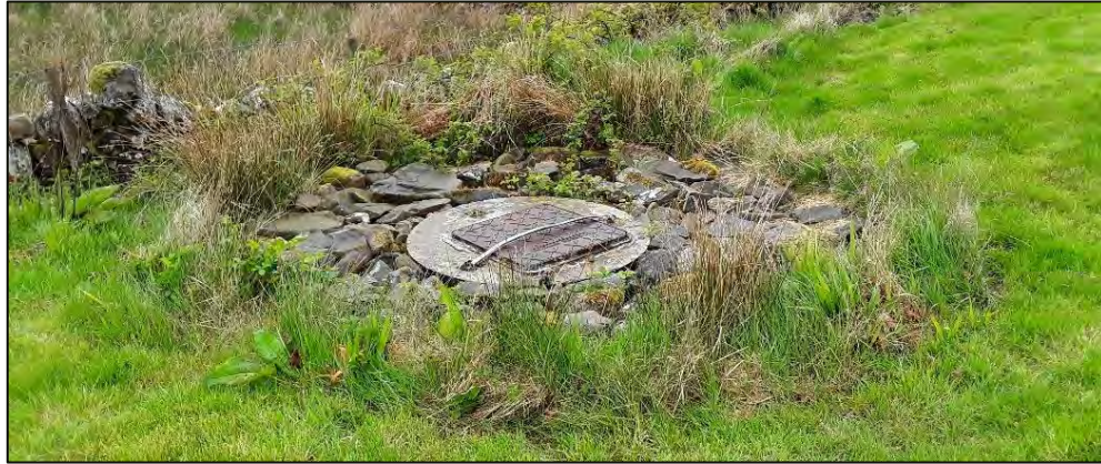
Photo 3: Capped spring source for Cot Cottage PWS and property
