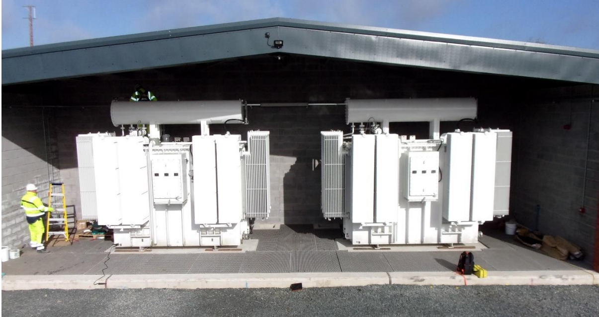
Figure 10. Semi-enclosed transformer bay showing mechanical completion of the two 17MVA transformers.
