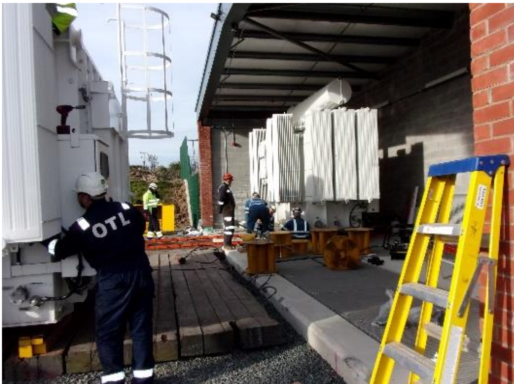
Figure 8. Photograph of transformers being slid into position at Llanfair PG substation. The farthest transformer can be seen with its fins and conservator fitted.
