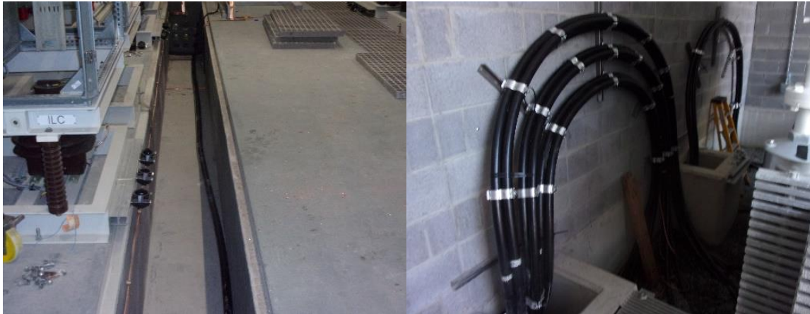
Figure 9. MV AC cable running from the valve hall trenches (left) to the transformer bay (right). Cables have been cleated in a trefoil arrangement.
