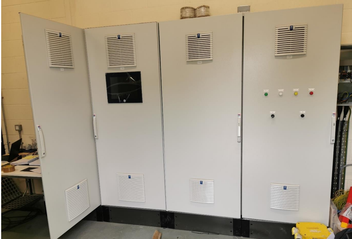
Figure 15 MVDC Station control panel showing HMI screen.
