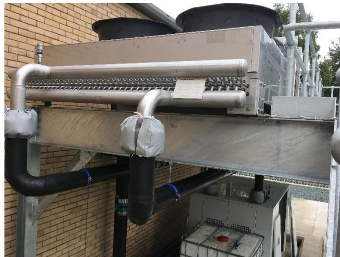
Figure 16 Heat exchanger located on gantry above the pump skid
