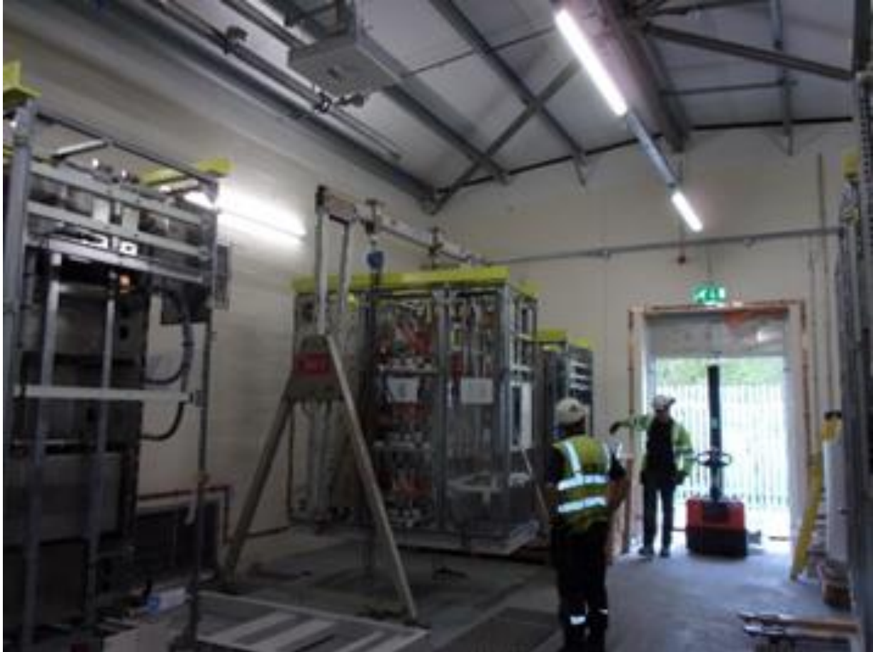
Figure 5. Photograph of a converter module before it's installed onto its base and post insulators.
