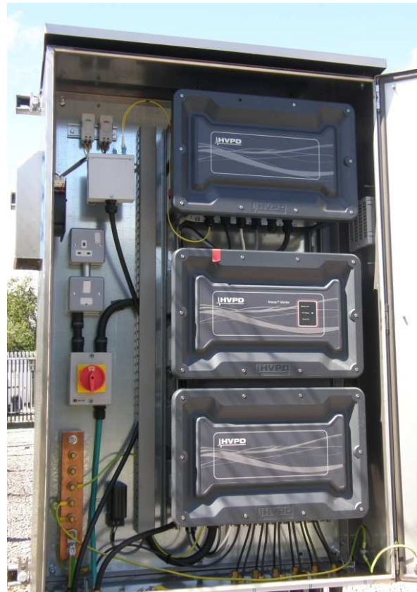
Figure 9. Kronos cabinet showing internal equipment..
