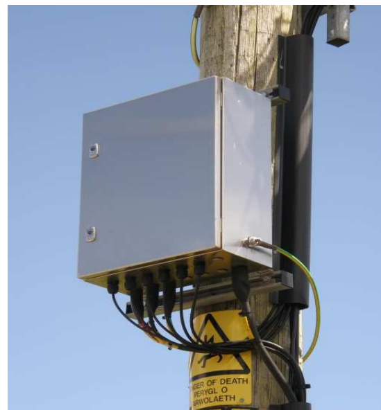
Figure 7. Local connection box mounted on termination poles.
