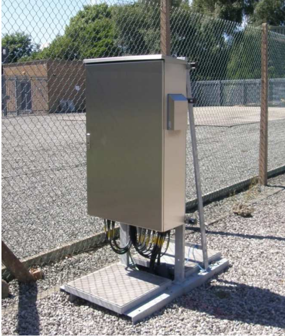
Figure 8. Kronos cabinet containing local data storage and power quality equipment.
