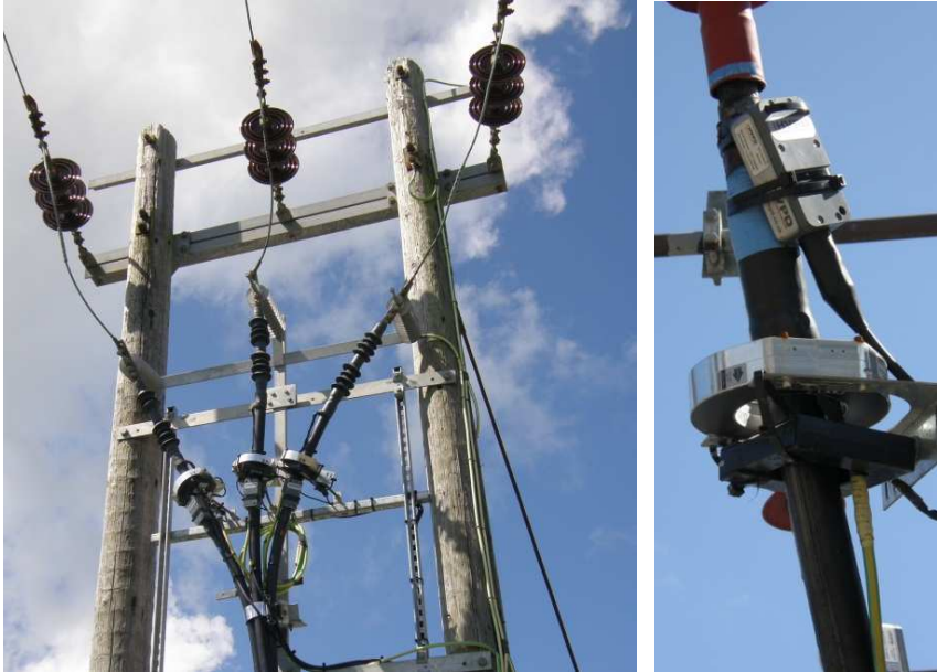
Figure 6. Cable terminations with HCCM sensors fitted.
