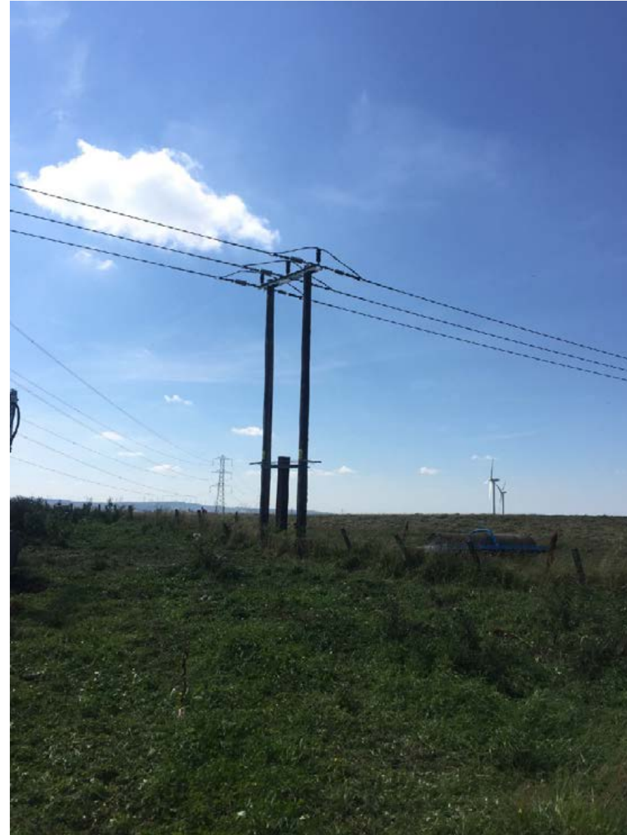
Typical Wood Pole (L36)
