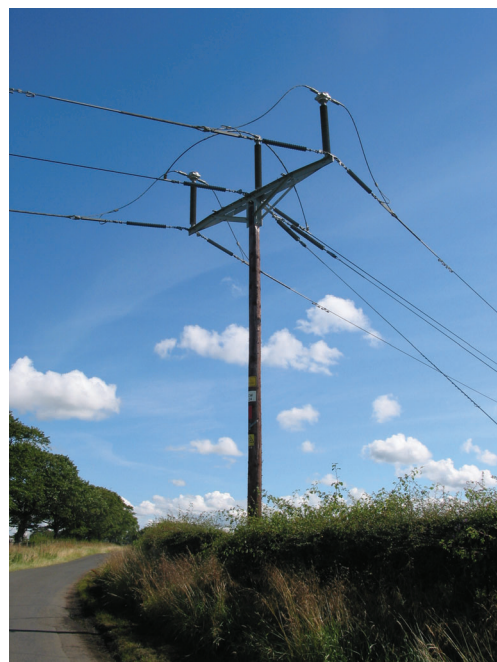
Trident single pole, vertical insulators
