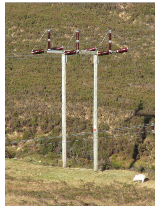
Trident 'H' pole straight-line pole
