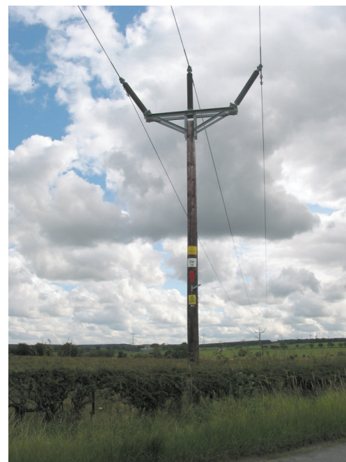
Trident single pole, 'trident' insulators
