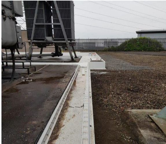
FIGURE 18 – AN EXAMPLE OF A TRANSFORMER BUNDED USING HDPE
