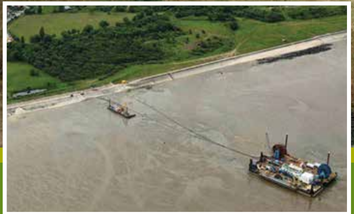
Marine cables will need to be installed in addition to underground cables
