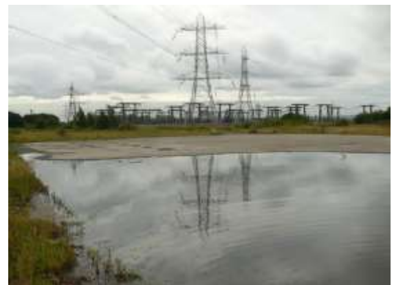
Figure 3.5: Existing substation at Kincardine, which contains an air insulated switcher (AIS).
