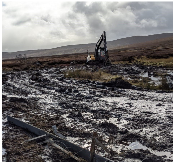
Damage caused by machine access to moor.
