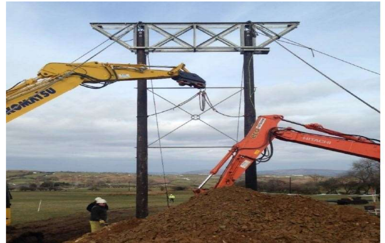
Figure 4.21: Erection of Wood Poles using a tracked excavator. This picture is for illustration only, the pole being erected is not a trident pole.
