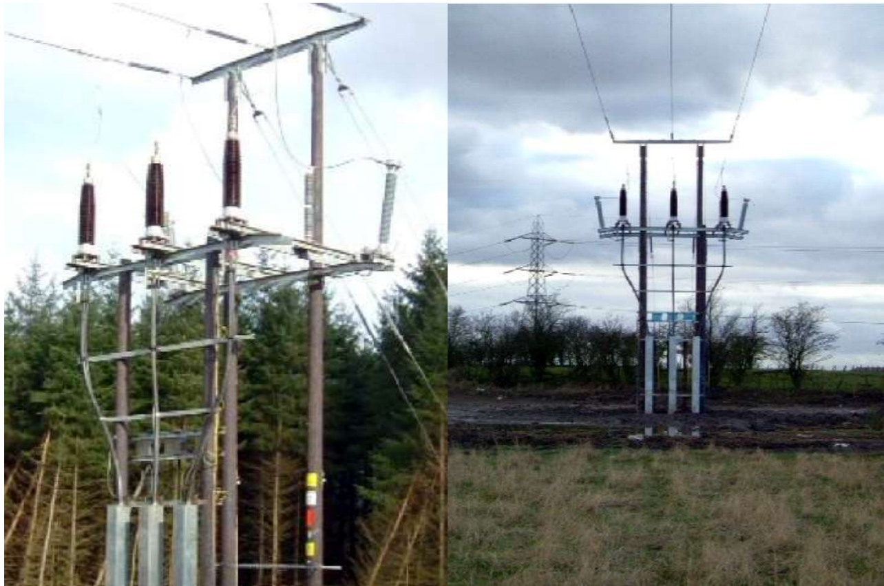
Figure 4.6: Typical pole mounted cable termination
