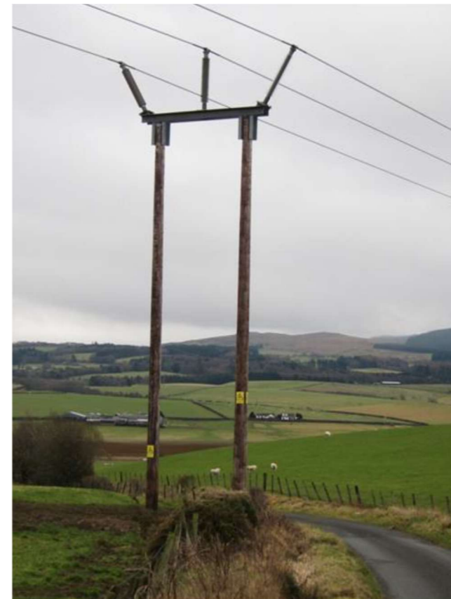
Figure 4.4: Typical trident 'H' pole
