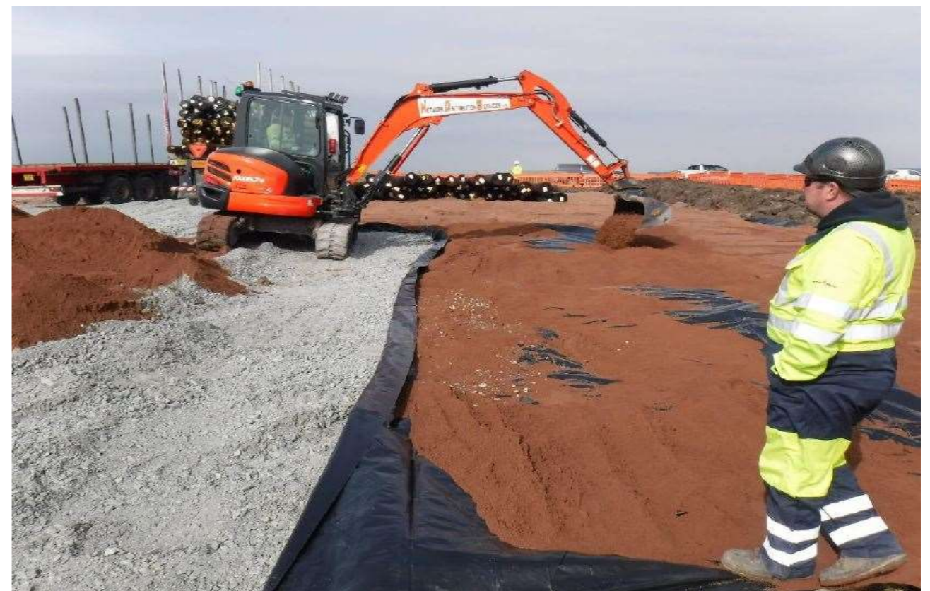
Figure 4.9: Typical pole storage on a hardstanding area, with a non-permeable membrane with sand to prevent leaching
