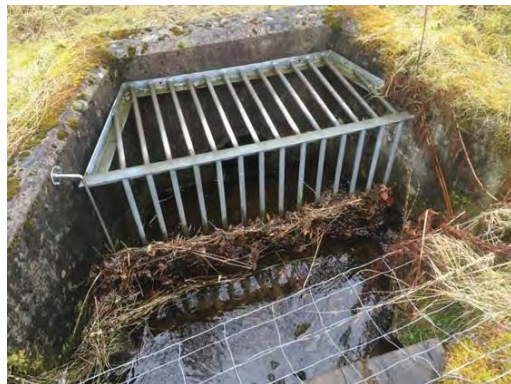
Figure 2: Pipe and screening present where watercourse enters the sub-station
