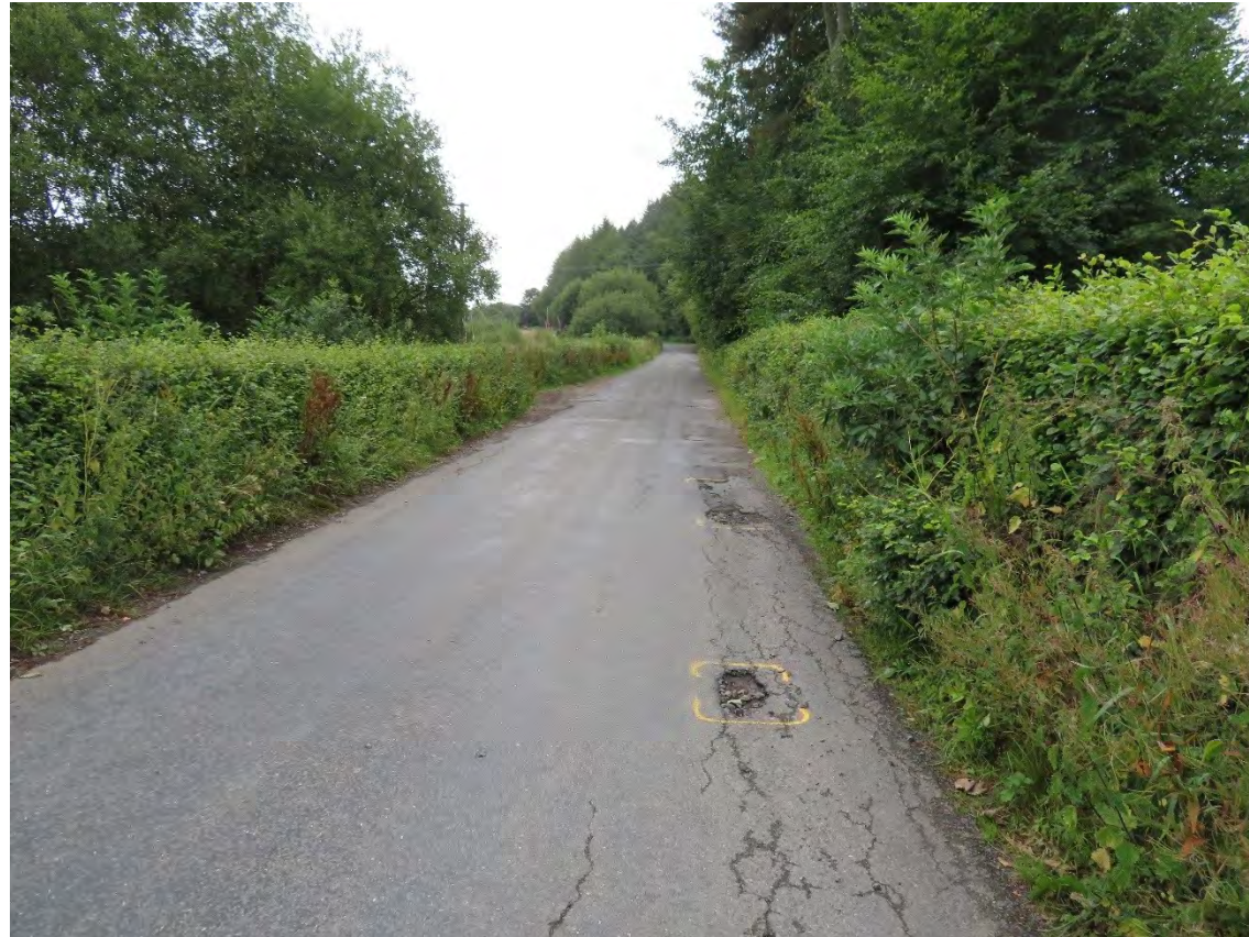
Figure 2-4: U2s Surface Edge Erosion
