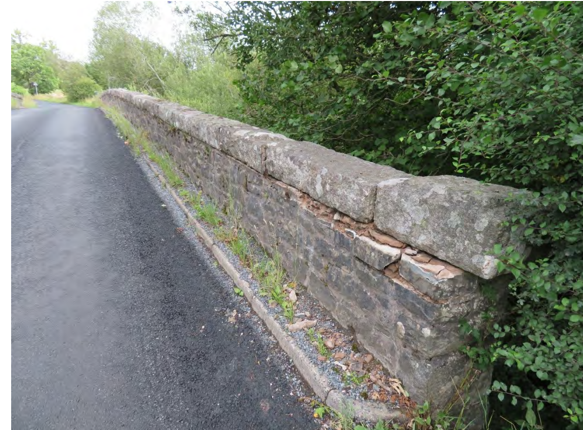
Figure 2-3: Coom Bridge Parapet Damage
