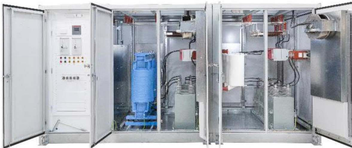
Figure 8. Typical arrangement of Enclosed Capacitor Bank
