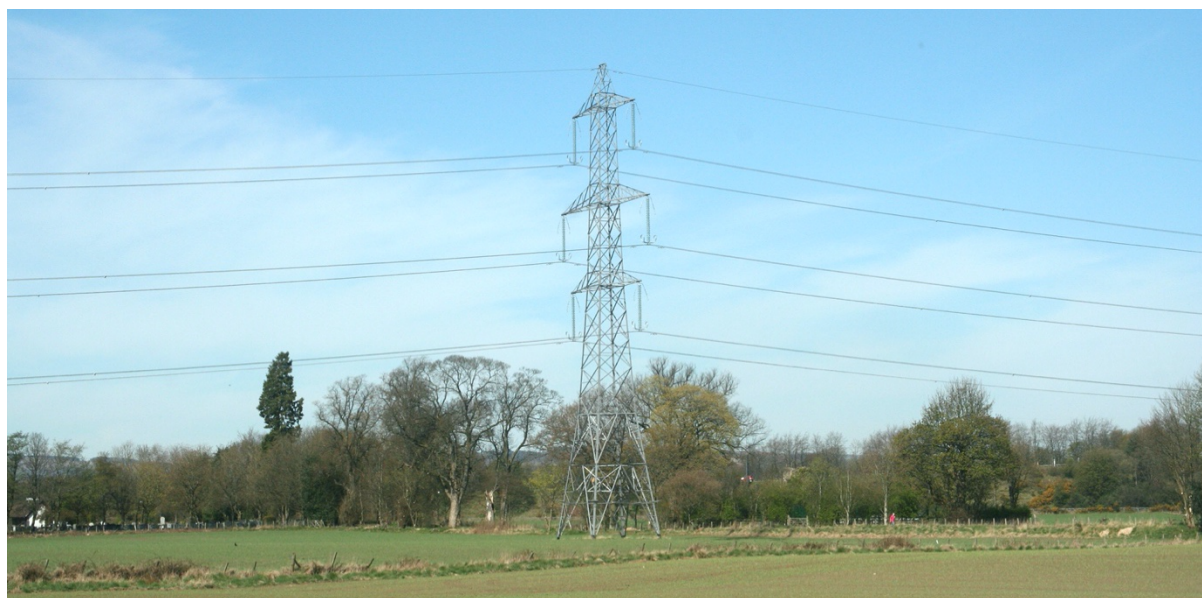
Figure 5 – A typical double circuit 275kV transmission overhead line
