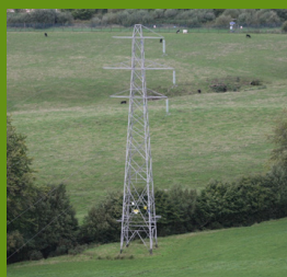
Single circuit steel lattice tower
