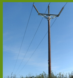
Typical Trident single wood pole
