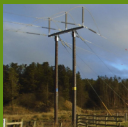
Typical double wood 'H Pole'
