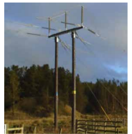
Typical double wood 'H Pole'
