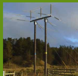
Typical double wood 'H Pole'
