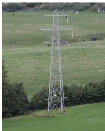
Single circuit steel lattice tower
