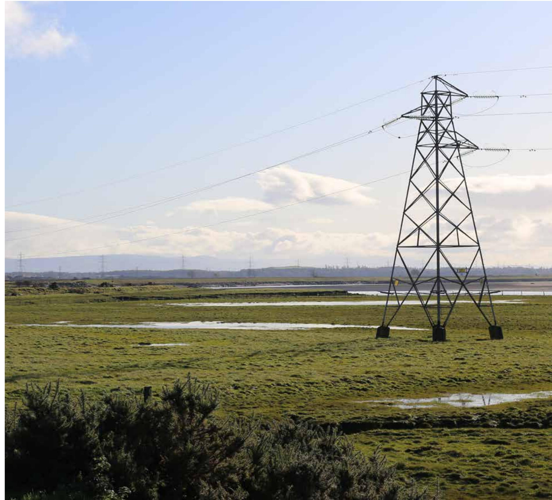
Photo 1: Tower T137A south of Gretna
