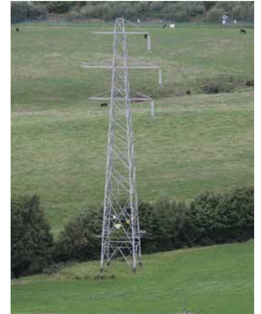
Photo 6: Single Circuit Steel Lattice Tower with conductors only on one side
