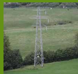
Single circuit steel lattice tower
