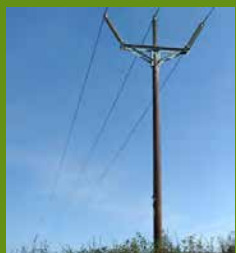
Typical Trident single wood pole
