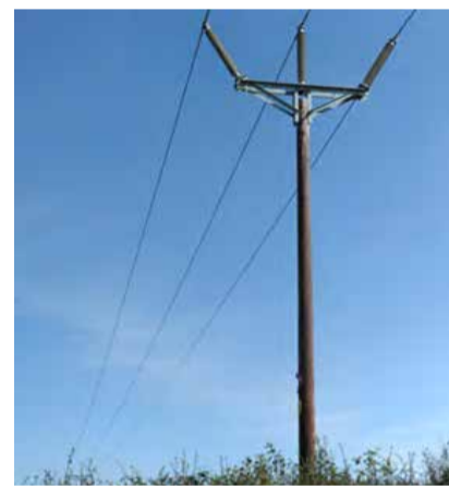
Typical Trident single wood pole
