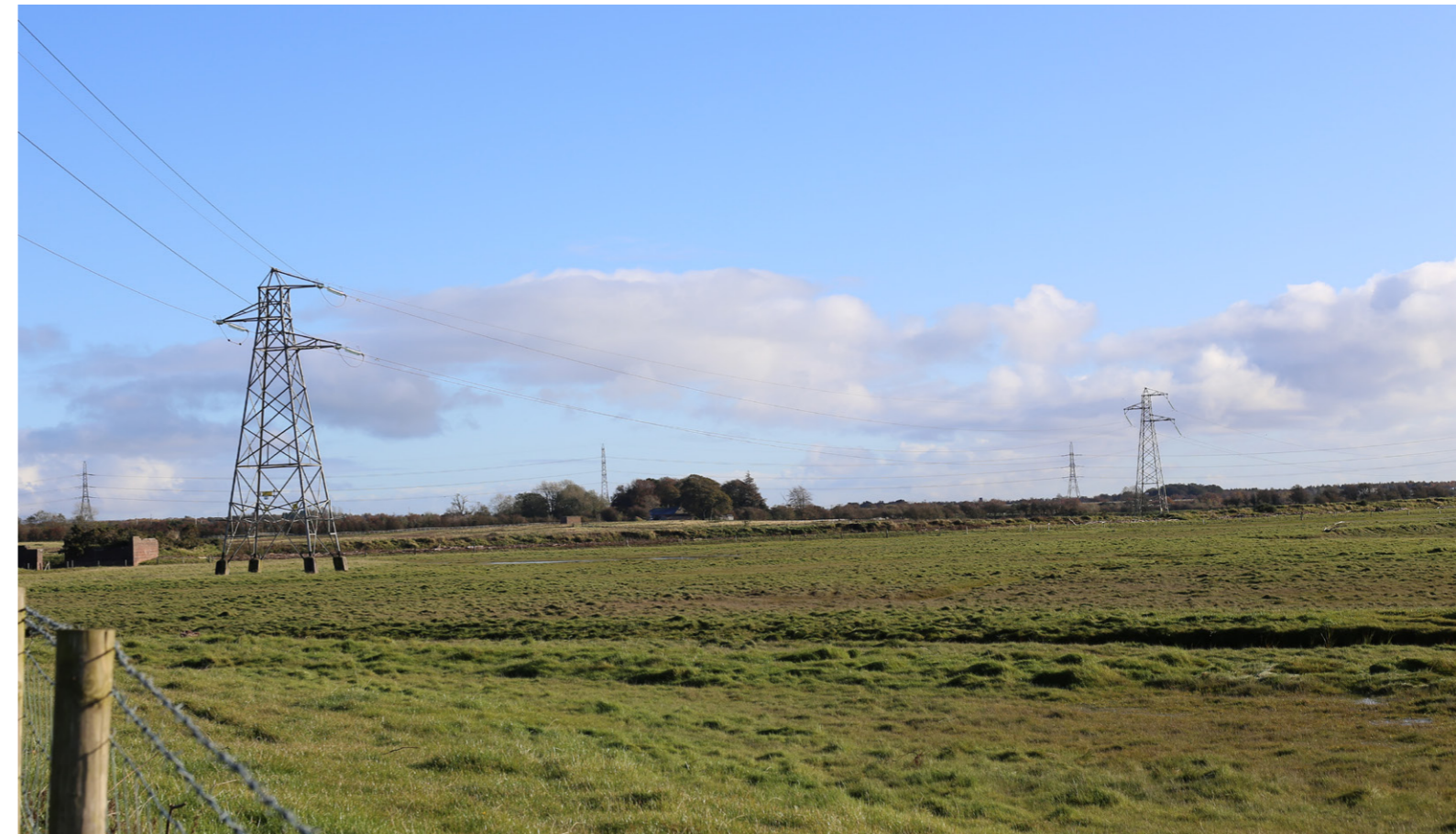
Photo 2: Existing steel towers on T Route
