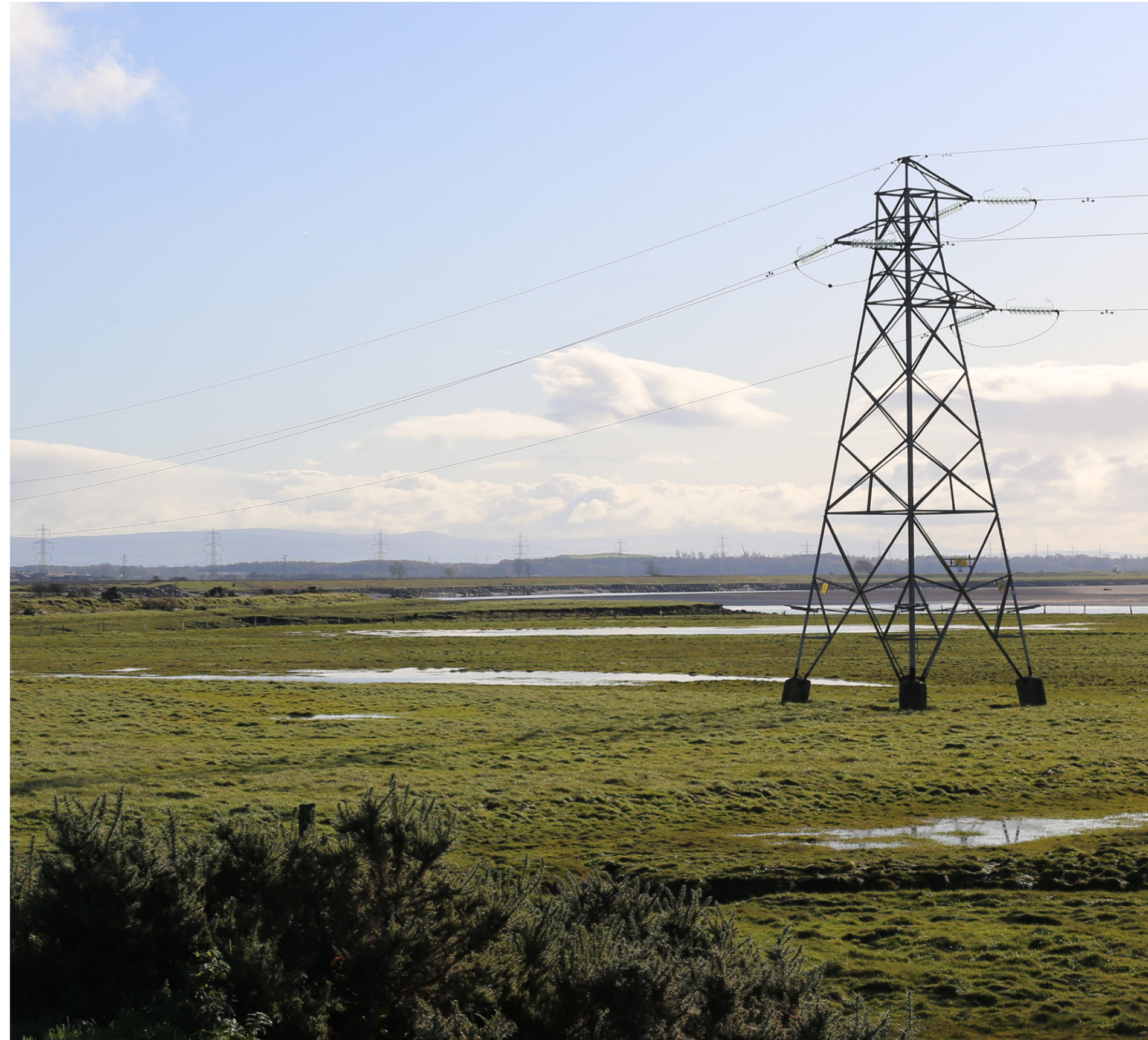
Photo 1: Tower T137A south of Gretna
