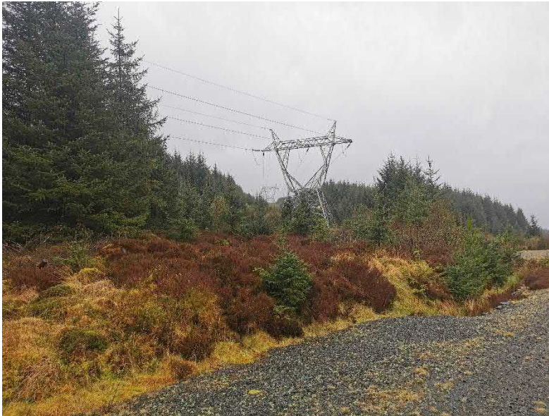
Photo 2-2: Facing south-west from Carrick Forest Drive along the existing “YY route” towards tower YY092 (to be retained) (Tower 2 type)
