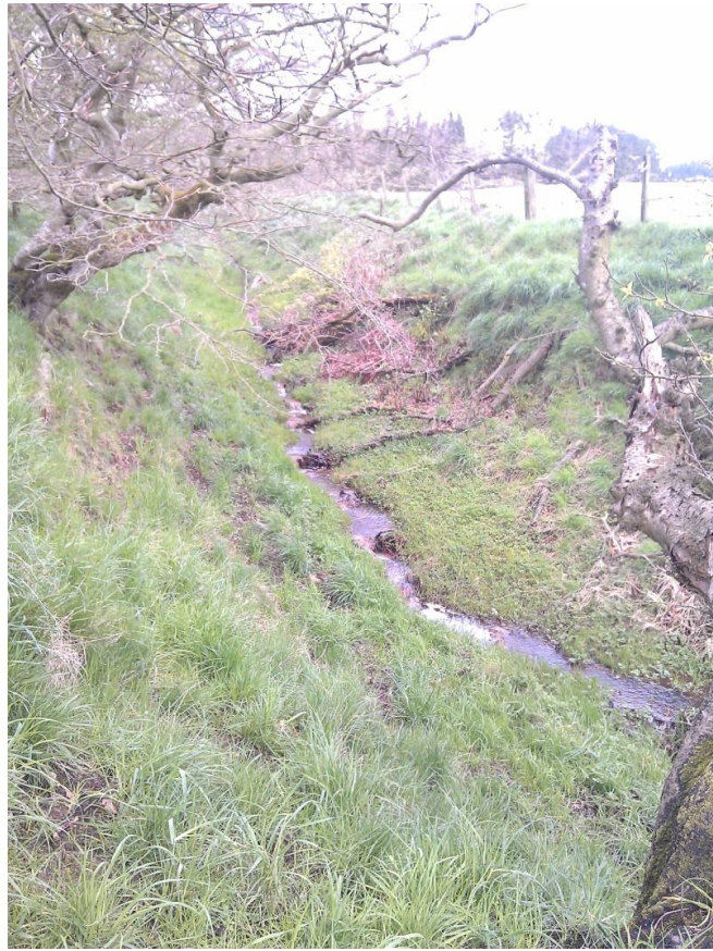
Plate 7.17: Brocklinn Burn tributary 1 upstream of the existing culvert crossing under the railway
