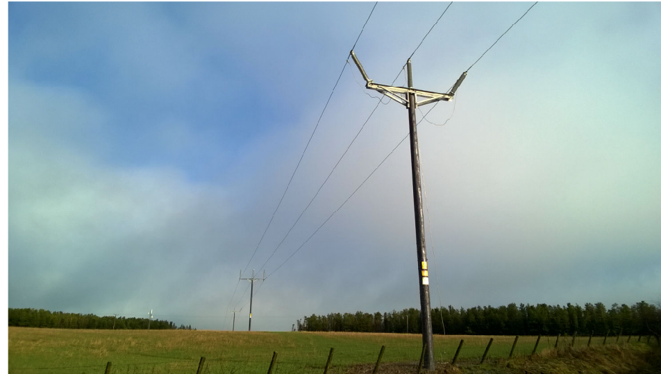
Trident Single Pole Intermediate (Foreground), Angle (Middle Ground)
