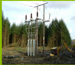
Terminal 'H' pole
