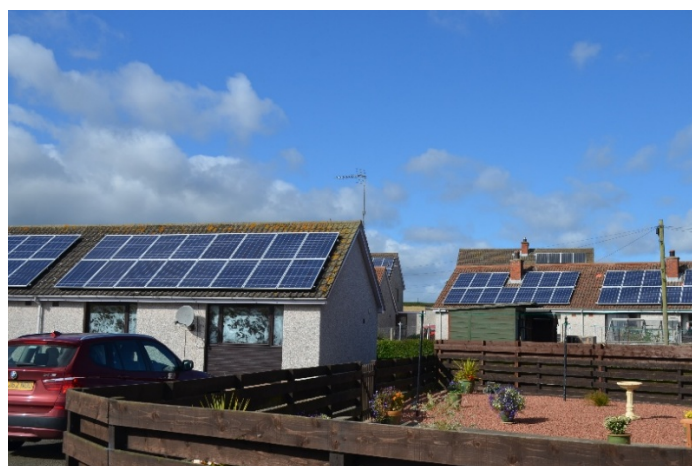
Figure 5: Installed PV panels
