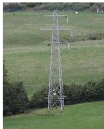
Single circuit steel lattice tower
