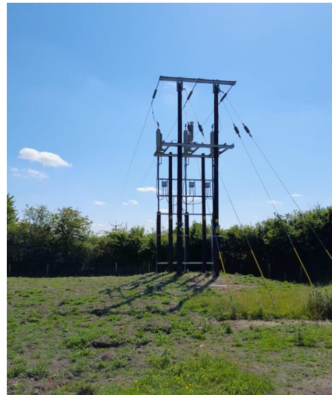
Photo 4.3: Example of typical terminal structures of a trident 132 kV OHL (SPEN, 2019)
