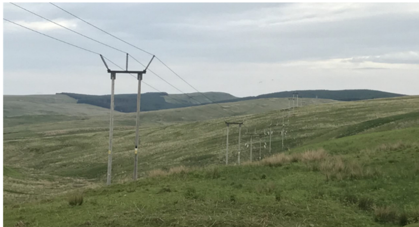
Photo 4.1: Example of a typical 132 kV H-pole trident OHL (SPEN, 2021)
