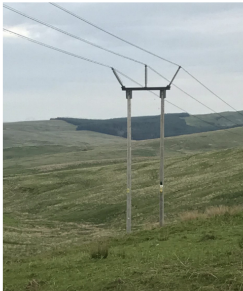
Photo 4.2: Example of a typical intermediate section of a trident wood pole supporting a 132 kV OHL (SPEN, 2021)
