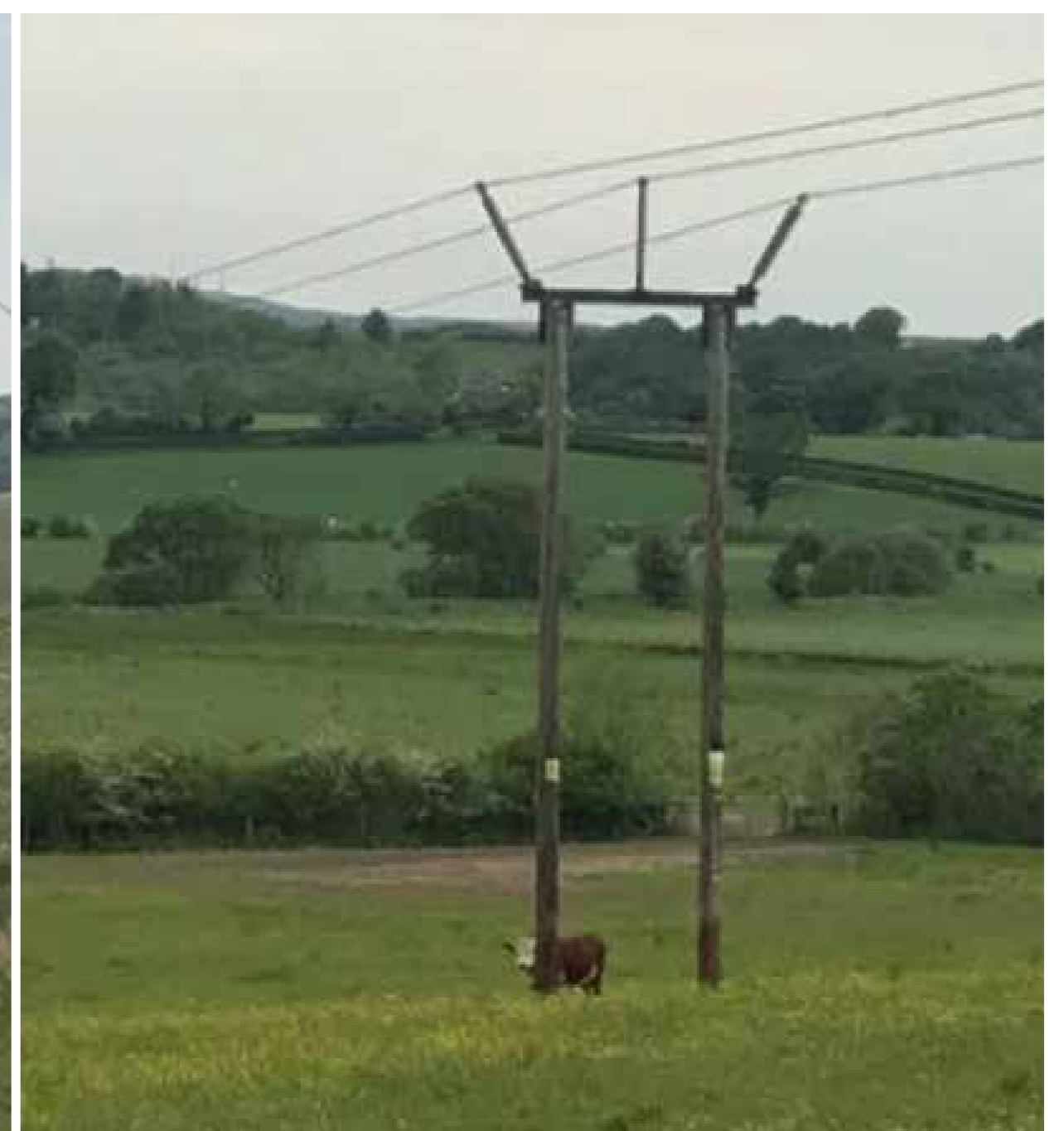
Example of a typical intermediate section of a trident double wood pole supporting a 132-kV OHL (SPEN, 2019)
