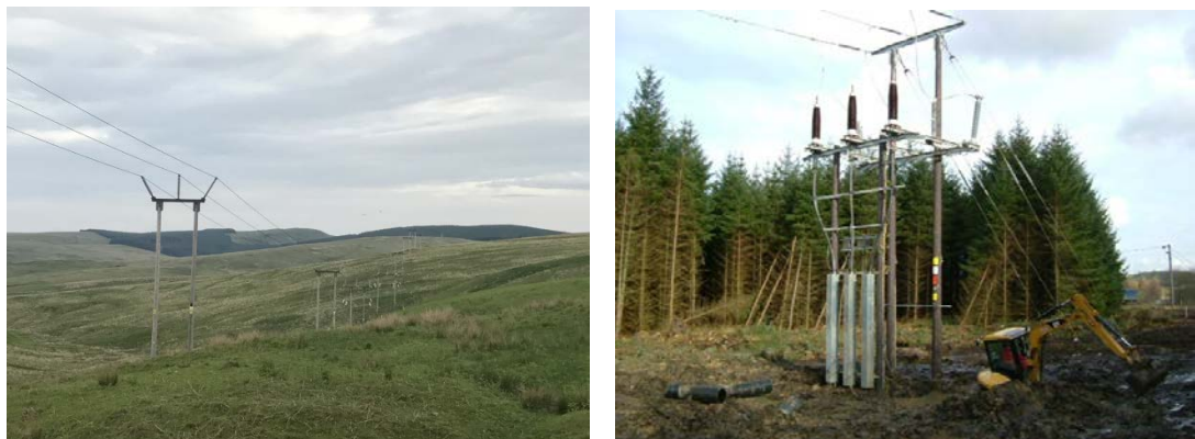
Figure 1.1: Example of a typical 132 kV H-pole trident OHL and terminal structure of a trident 132 kV OHL (SPEN, 2021)
